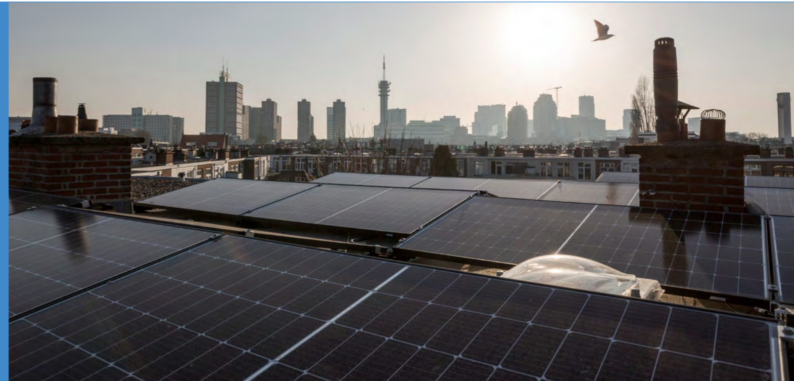
Figure 6: A solar roof with The Hague's skyline in the background
