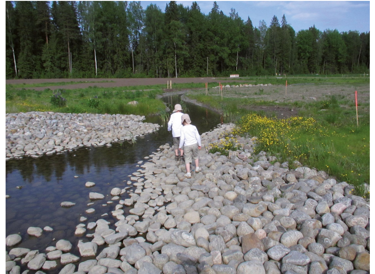
Image 53. Natural drainage systems are being actively developed in Tampere. For example, one of the largest drainage areas in Finland, which also serves as a recreational area for residents, has been built in Vuores. Water quality and flow are monitored by automatic measurements throughout the year. Measurements provide information on the ability of the current drainage system to purify drainage water and to reduce flows. The Urban Nature Labs project piloted urban drainage water management through nature-based systems in collaboration with city residents throughout the city, for example in Hiedanranta. Image: City of Tampere.
